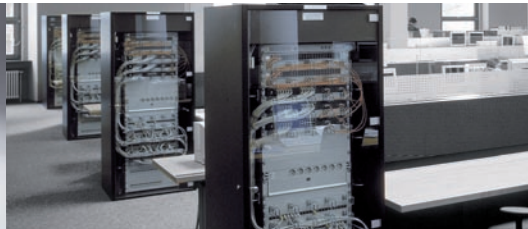
Individual Cool-Rack cabinets
