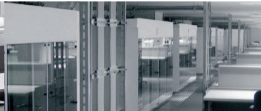
Cool-Rack connected to four-way units
